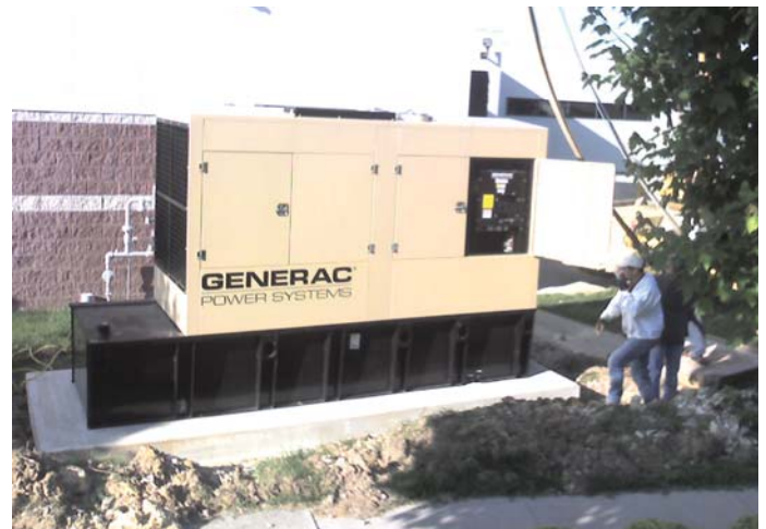
The PSRS Backup Generator
